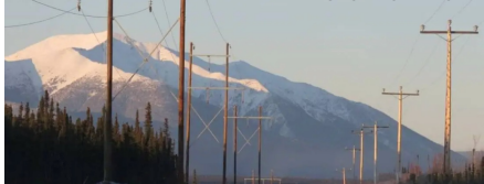
YUKON POWER GRID
